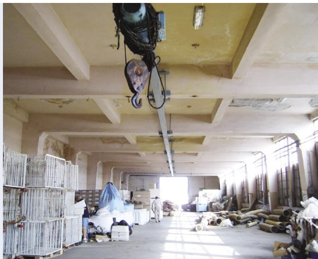
Bulgarian facility before Installation
