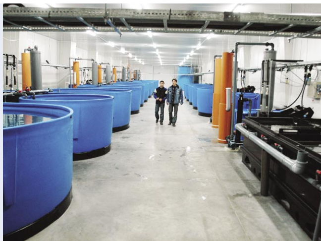
Bulgarian facility after Installation
